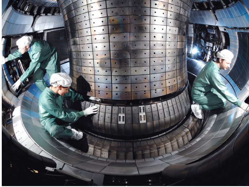
Figure 1.1: Installation work inside the plasma vessel of the Tokamak reactor at IPP Max-Planck Institut für Plasmaphysik. The transformer coil is situated behind the column. The plasma vessel is surrounded by the main and the vertical-field coils ( http://www.ipp.mpg.de/16208/einfuehrung ).
